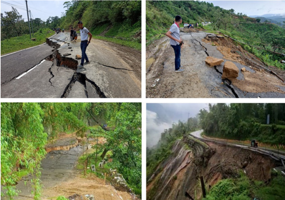
Fig 1B: Specimen photographs of eroded section of highway along the Maibong and Ditokcherra stretch (Sources ASDMA).
