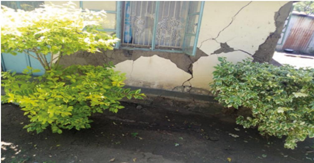
Plate 1: Destruction of a house due to effects of flood in Magina (Source: Author May, 2019)
