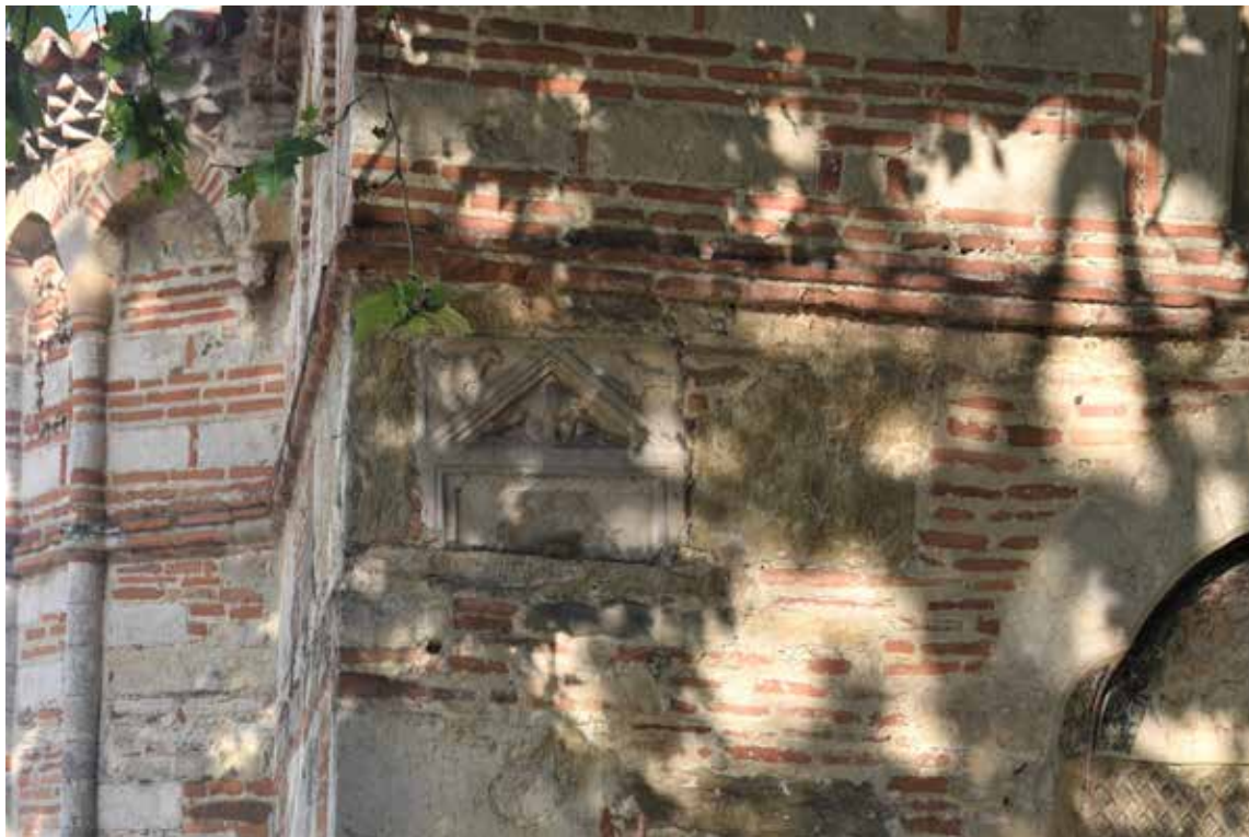
Figure 2a. Detail of the west facade of the Church of the Assumption of the Blessed Virgin Mary, Smederevo (photographic documentation of the Institute of Archaeology, Belgrade).
