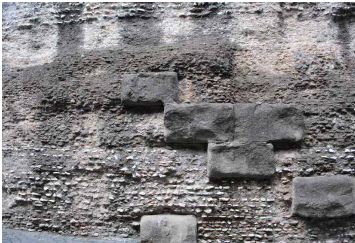
Fig. 5. Opus caementicium foundation of the Hadrian Mausoleum in Rome (today's Castel Sant'Angelo) in Rome (mid 2 nd century AD) (Dilaria in press).
