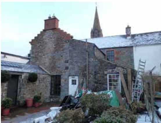
Fig. 11. Archbald Moffat House, Moffat, two years after repointing with NHL 5.0 mortar (photo by N. Copsey from Copsey 2019a).
