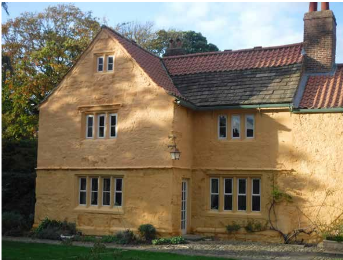
Fig 23. Hot limewashed exterior, reinstating original coating and pigment (iron sulphate). Bishop Burton Old Hall. Limewash offers moisture buffering and capillary activity across the whole surface area of building elevations (photo by N. Copsey).
