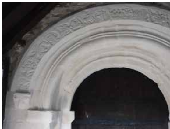
Figs. 18a. and 18b. Hot lime sheltercoat to a 12 th century doorway (with recycled Roman columns), St Michael's Church, Foston, near York (photos by N. Copsey from Copsey 2019a).
