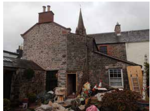
Fig. 12. Archbald Moffat House, Moffat, two weeks after repointing with a hot mixed air lime mortar and after 12 hours of rainfall (lean-to on the right still retains NHL pointing) (photo by N. Copsey).
