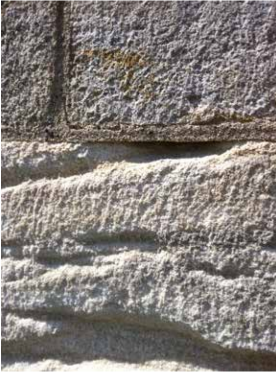
Fig. 15. Pennine sandstone, 20 years after repointing with St Astier 3.5 mortar. Salt-induced decay of the sandstone; no sacrificial behaviour in the mortars, Studley Royal, North Yorkshire (photo by S. Baxter from Copsey 2019a and 2019c).
