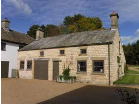
Fig. 10. A humbler building of similar geology, pointed with hot mixed air lime mortars, Pockley, North Yorkshire (photo by N. Copsey from Copsey 2019c).
