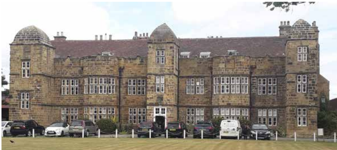
Figs. 8 and 9. Marske Hall; porous Jurassic sandstone' Repointed with NHL. Winter and summer, the latter image taken after five months without significant rainfall (photo by N. Copsey).
