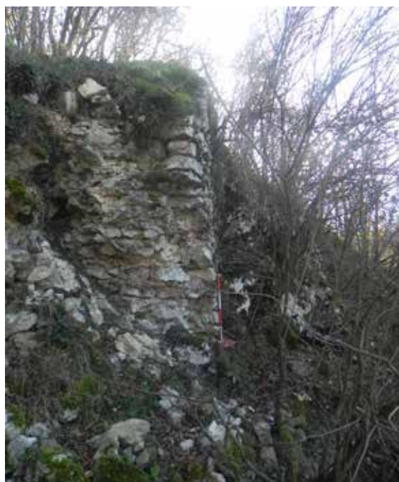
Fig. 11 Damage to the defensive wall in the middle part.
