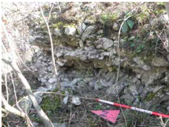
Fig. 13 Damage to the southern part of the defensive wall at the external face.
