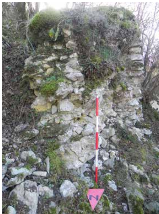
Fig. 8 Damage to the defensive wall on the northern part.
