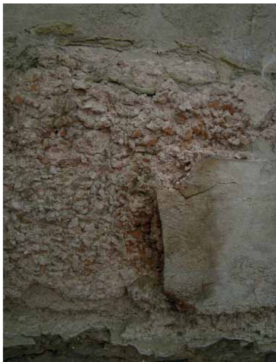
Fig. 12 Rendering layers of Viminacium thermae with brick in the form of large fragments.
