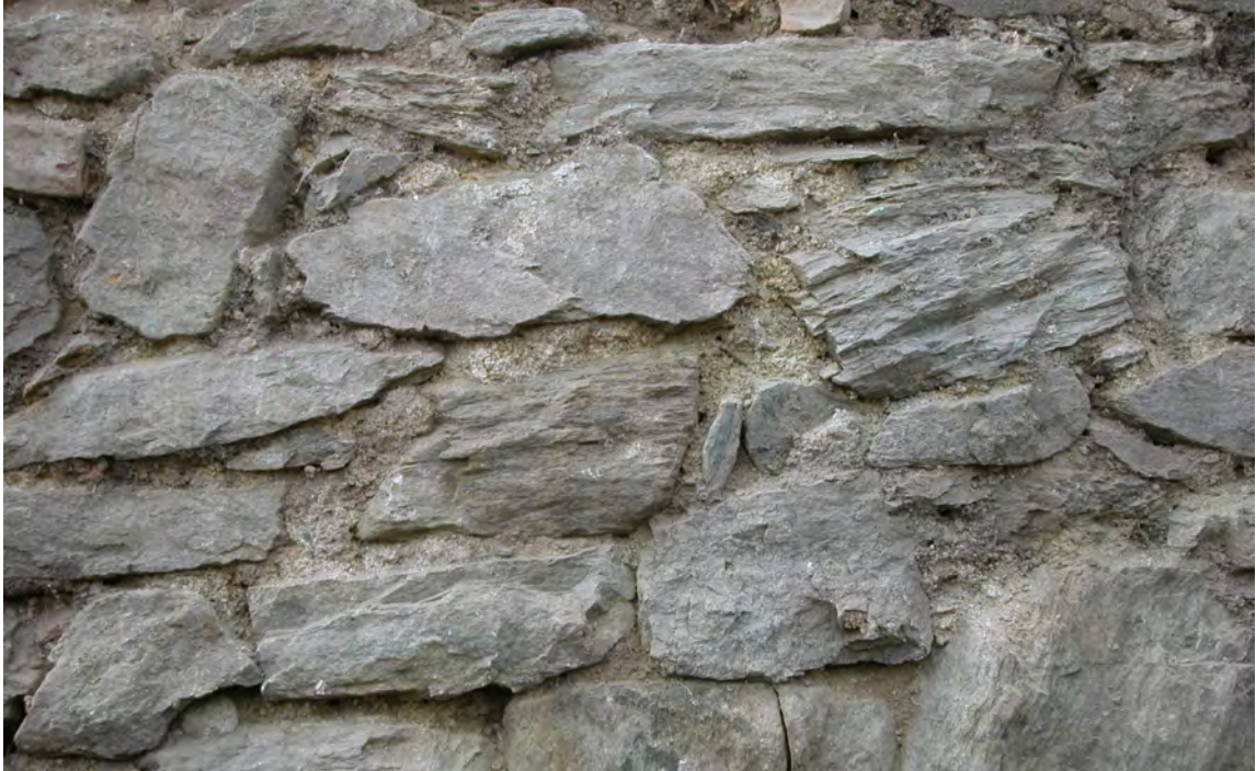
Fig. 31 Opus incertum in the walls of Viminacium thermae. Photo by the author.
