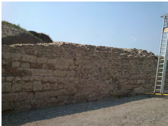
Fig. 28a Arched wall of the amphitheatre arena with visible repairs. Photo by the author.
