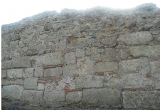
Fig. 28b Arched wall of the amphitheatre arena with visible repairs, details. Photo by the author.
