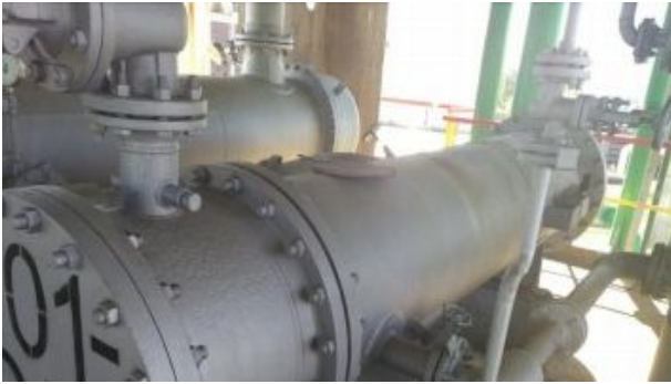
Fig.2. The condenser considered in the case study
