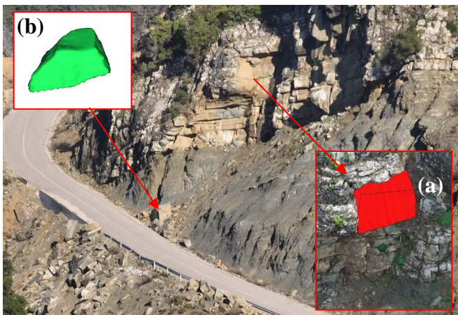
Figure 8 The northern section of the slope clearly reveals the origin of rockfalls in Type III flysch above Type VIII. The failure mechanism is evident, characterized by the undercutting of the sandstone as a result of the differential erosion of the underlying siltstone. a) the main rockfall source with 13 m 3 volume, measured by digital reconstruction of the detachment geometry, and b) a 6.5 m 3 block from this detachment, located on the slope side.
