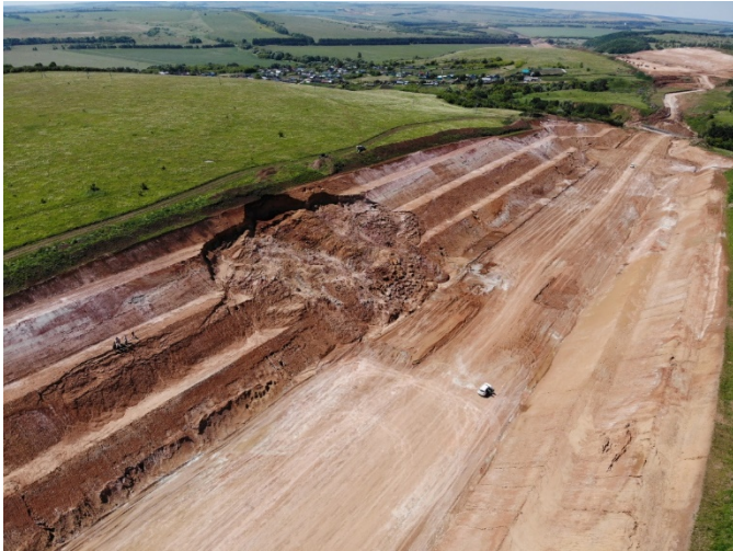
Figure 1 Sliding landslide at the construction site of the M-12 highway.
