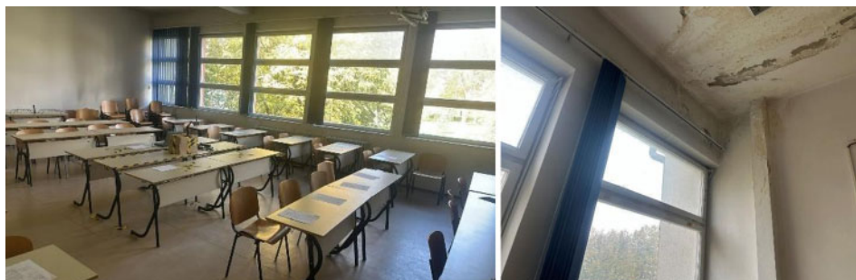
Figure 1: Lecture room at the FPES, position of the device for measuring air quality parameters (picture on the left), and the appearance of moisture on the ceiling due to a leaking roof (picture on the right)
