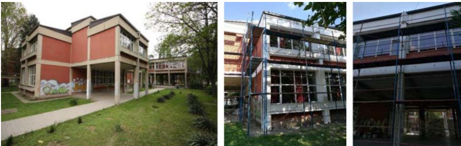
Figure 3 (left): High School “Orce Nikolov”– original façade, source: https://marh.mk/ ; Figure 4 (right): High School “Orce Nikolov”– reconstruction, source: https://marh.mk/
