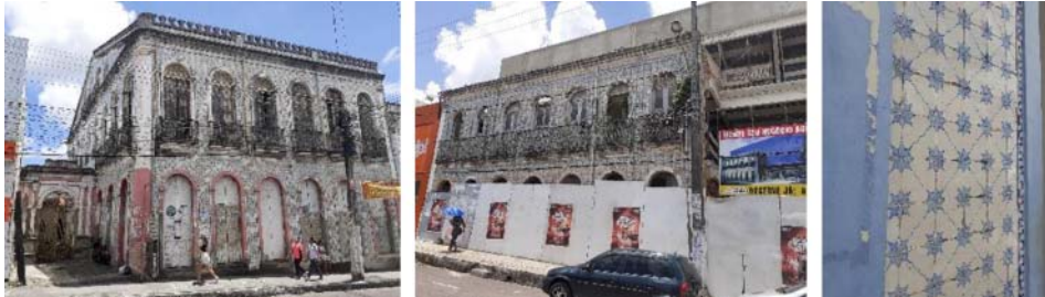
Figure 5: Houses and Townhouses Covered with Portuguese Tiles, Estância, Sergipe, Brazil. (Photos: Janaina Mello, 2021).
