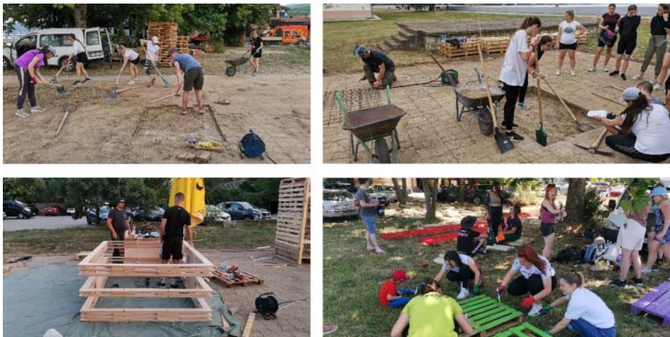
Figure 3-6: The building camp was organised into four days: Day 1 – dirt and sand excavation; Day 2 – armature reinforcement and concrete work; Day 3 – finalising finish; and Day 4 – paint work and final arrangement (Author: M. Obradović).
