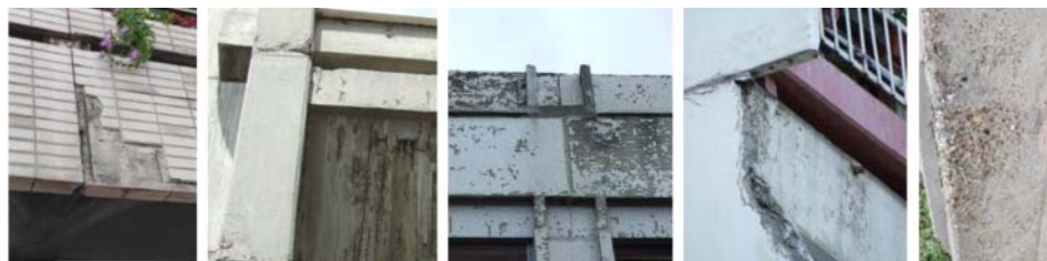
Figure 3: Diverse types of façade damages
