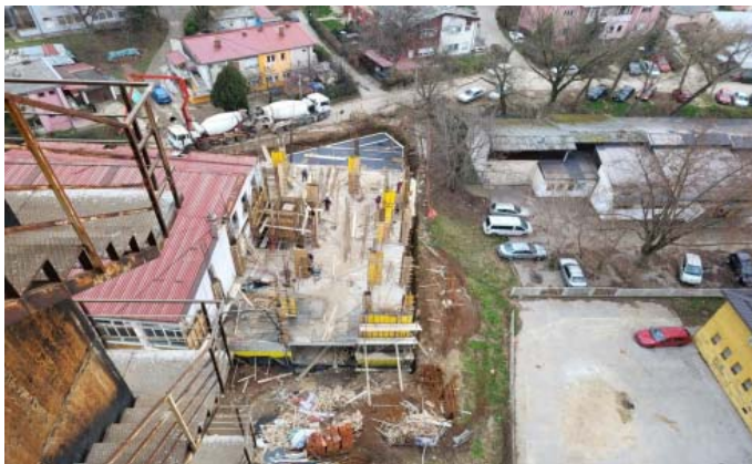
Figure2: a six story building is being built on a parking lot (source author)
