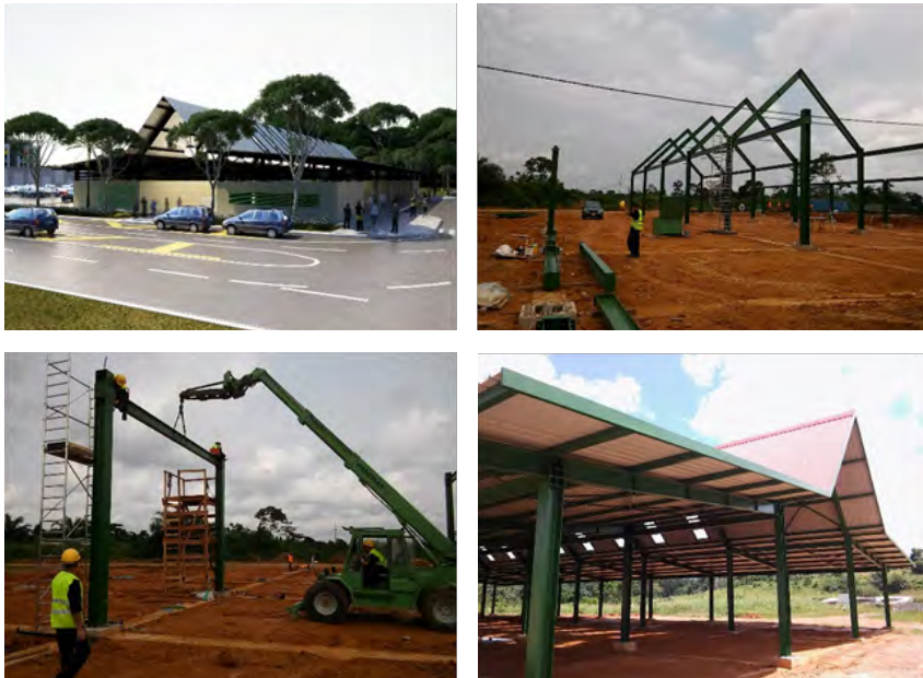
_ Figure 5: 3D render of the Okolassi market, construction phases and assembled structure.
