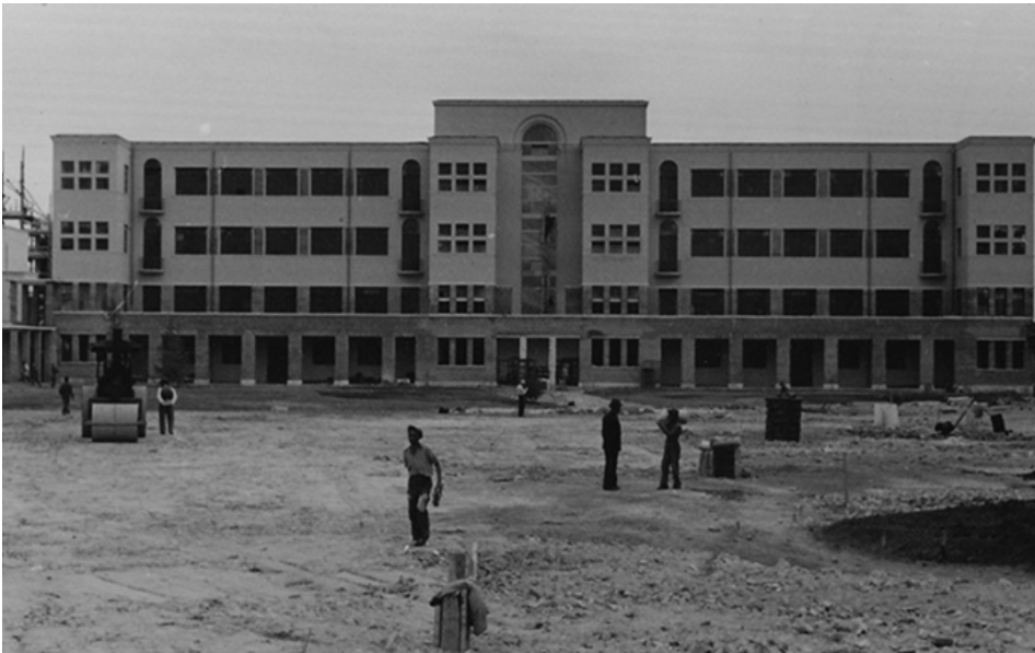
_ Fig. 3. Roman Institute of San Michele, buildings under construction, source: Alberto Calza-Bini private archive.
