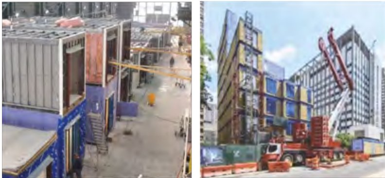
_ Figure 3: Fabrication and stacking of the steel framed modules of the Carmel Place building. (Source: Carmel Place Innovative Practices for Healthier Homes, A Case Study , 2019)
