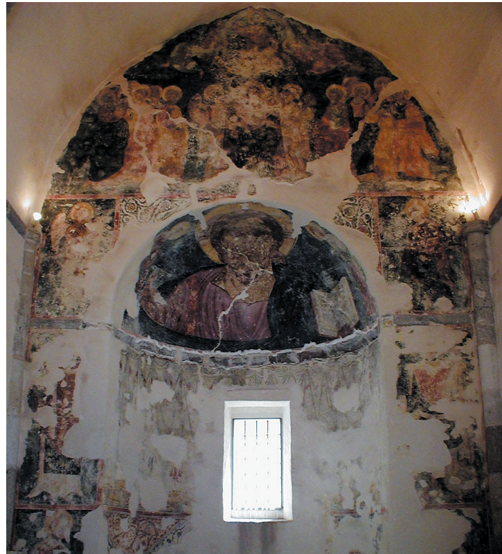
Fig. 10 View of the eastern wall and the apse, after the finished painting and conservation works
