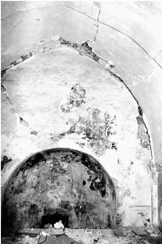
Fig. 9 Interior of the church, view of the eastern wall before painting and conservation research
